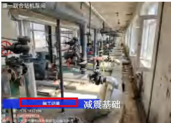
联合站站内机泵
