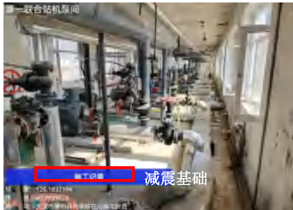
联合站站内机泵
