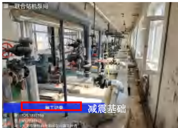
联合站站内机泵
