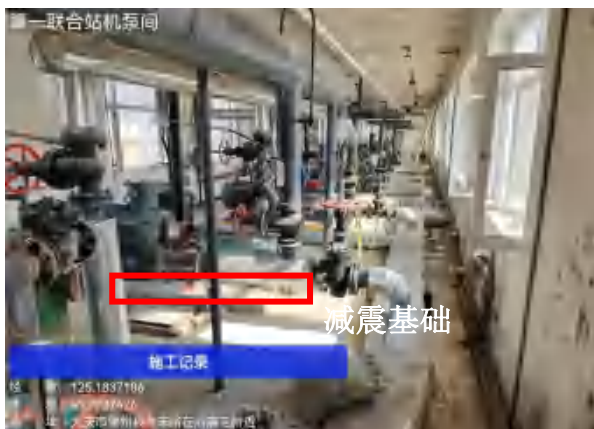
联合站站内机泵
